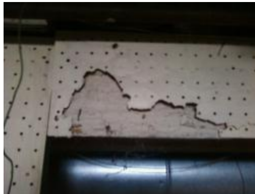
Termite Damage to basement pegboard
