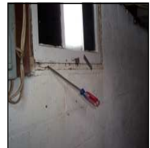
Hidden termite damage in basement window frame.
