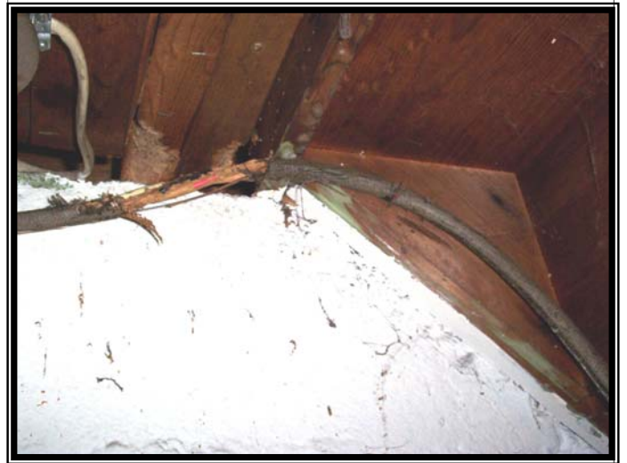
Gnawed Wires Beneath Basement Stairs
